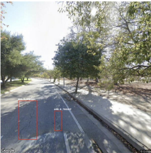
Fig. 2. Road damage detected by the YOLO model [1].
